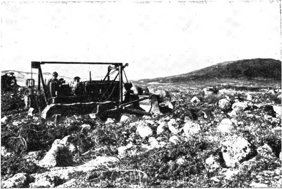
① Start of operations. Boulder clearing from natural gravel foundation. Leveling course of granular material required to provide uniform bearing for steel landing mat.
